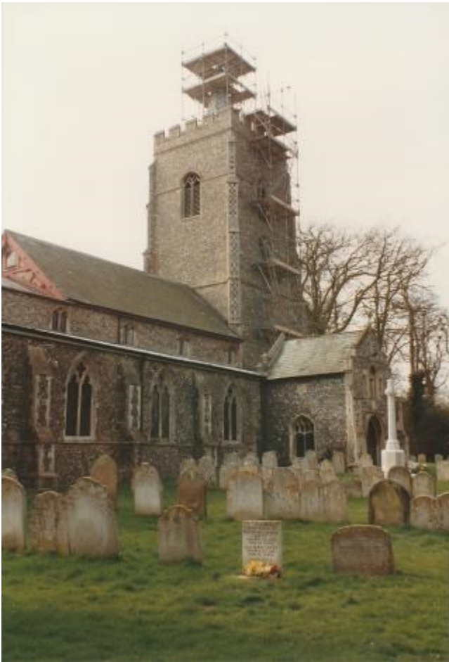
The repair/replacement of the steeple when the work took place in April 1993
